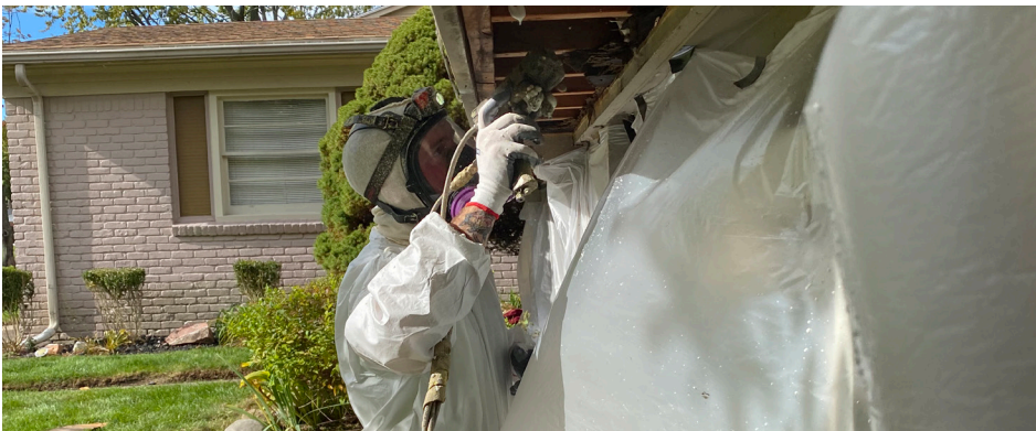
An installer with Ecotelligent Homes installs spray foam around the perimeter of the upper level, which cantilevers over the lower level.
