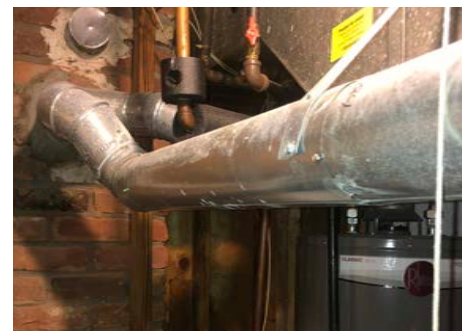
The attics, walls, and basement all had minimal insulation and no air sealing.
