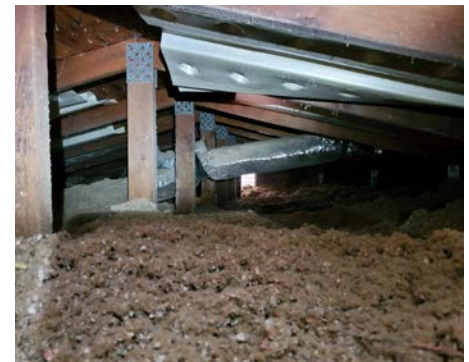
The upper attic was air sealed and insulated to R-49. New six-foot baffles facilitate attic ventilation.
