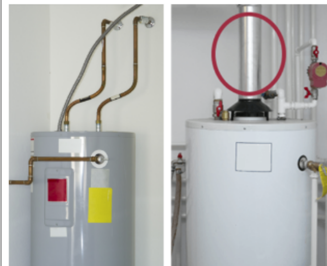
Figure 1: Conventional electric water heater without flue on left and gas water heater with flue on the right (exhaust flue circled in red).
