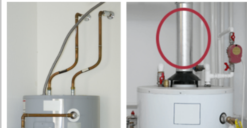
Figure 1: Conventional electric water heater without flue on left and gas water heater with flue on the right (exhaust flue circled in red).
