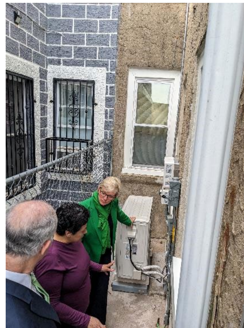
Sec. of Energy Granholm and Sen. Casey observing heat pump and solar installations at the BTL home
