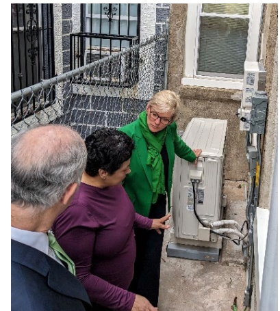
Photo caption: Senator Casey, Secretary Granholm, and Nancy with her new heat pump and rooftop solar system.
